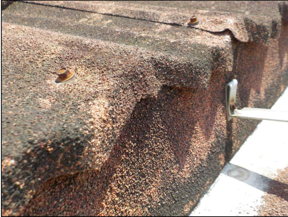
Typical condition of the coated metal r-panels
